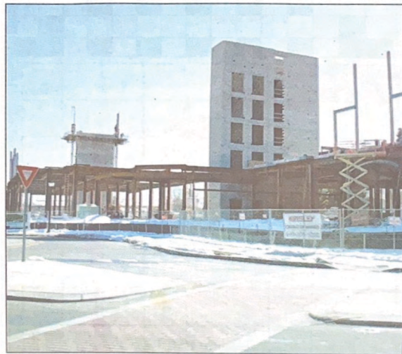
The construction at the circle on Rt. 322 is underway for an expected completion during the second half of 2011. The project is a large part of the revitalization of the Rowan University Honors program. - Staff photo/ Sarah Wecht
